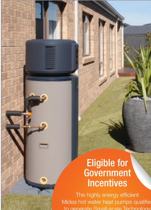
170L Installed Unit
